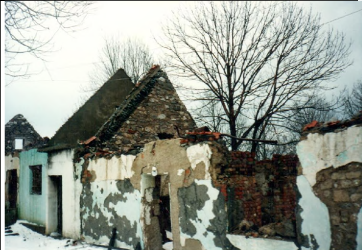
Buildings in Croatia showing war damage Photo provided by Bethan Mowat
